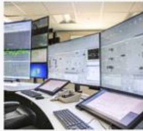
Industrial Process Control
