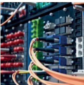
STRUCTURED CABLING SYSTEMS
