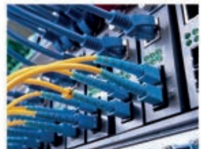
STRUCTURED CABLING SYSTEM
